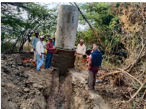
c. Over head tank for lift irrigation system
